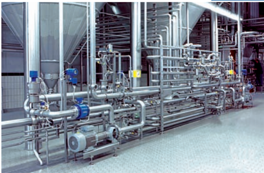
Hefetankanlage / Yeast tank system
